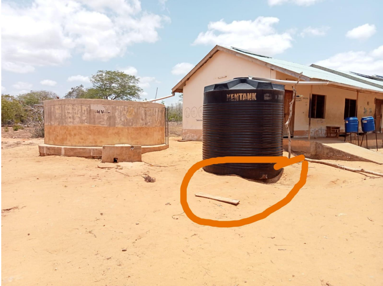
Figure 3. Baraka-Jembe School tanks 4 and 5
