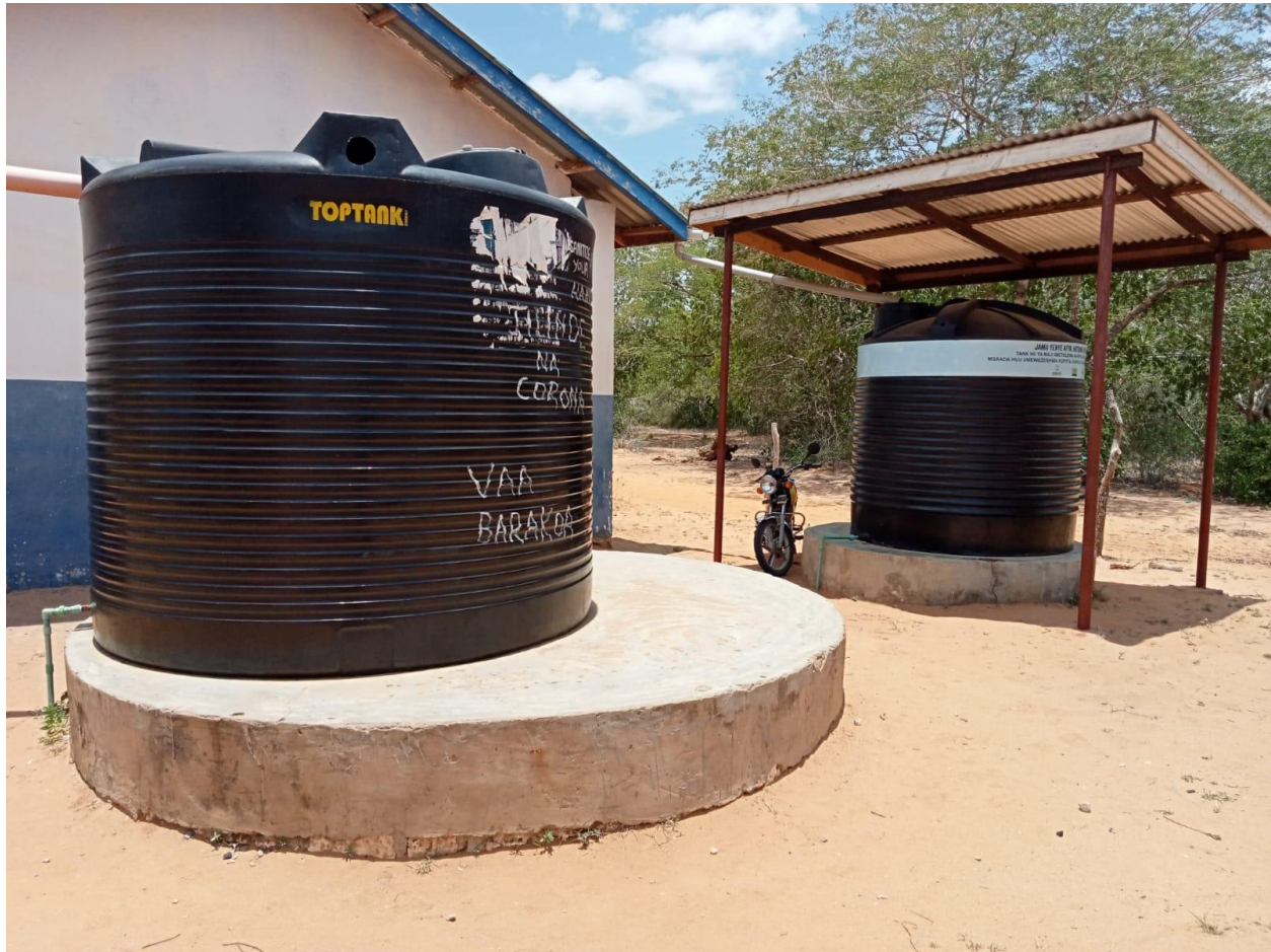
Figure 2. Baraka-Jembe School tanks 1 and 2
