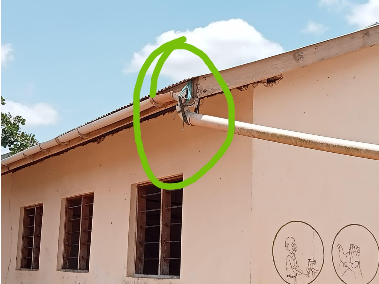
Figure 4. Baraka-Jembe School gutters failing
